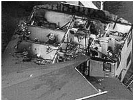
The roof of building J after the blaze.
