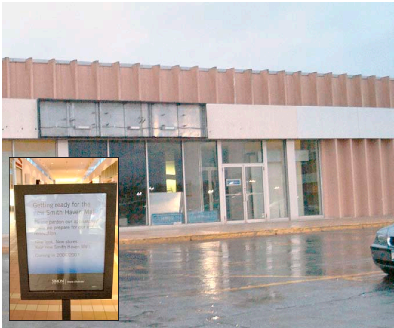
Sears entrance looks barren as small stores are being moved out to make way for new ones. Inset: a pardon our appearance sign, explaining the new renovations at the mall.
