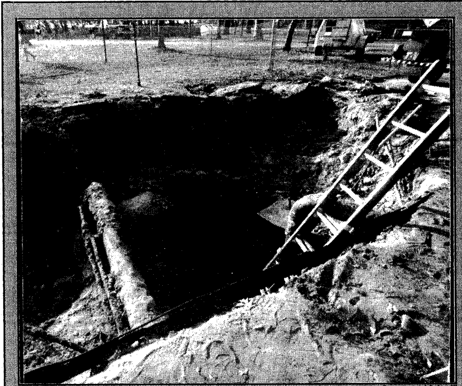
Source of steam leak outside of Gray College in Mendelsohn Quad that University officials say caused the short-circuit in the two electrical feeders.
