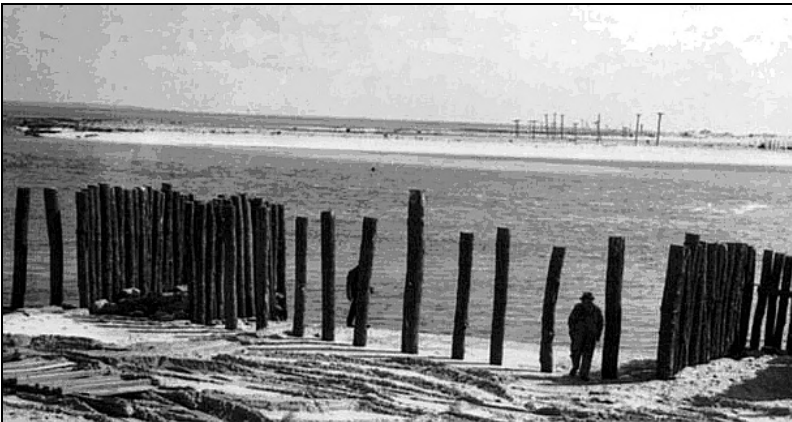
WPA project to replenish the banks of the Shinnecock Inlet. Note scale of thirty foot piles used in the project with ten foot lengths exposed 1939. Courtesy of the National Archives and Records Administration II, College Park, MARYLAND
