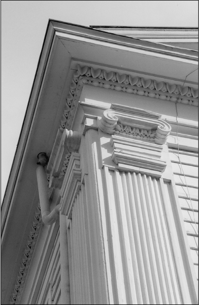
A view of a corner of Deepwells showing the intricate hand carved detailing on the Corinthian column and the overhang trim.
