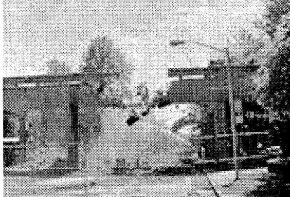
Courtesy of fsnt.gis.sunysb.edu/FDC The bridge connecting the Melville Library and the Union was demolished after many years of structural difficulties.
