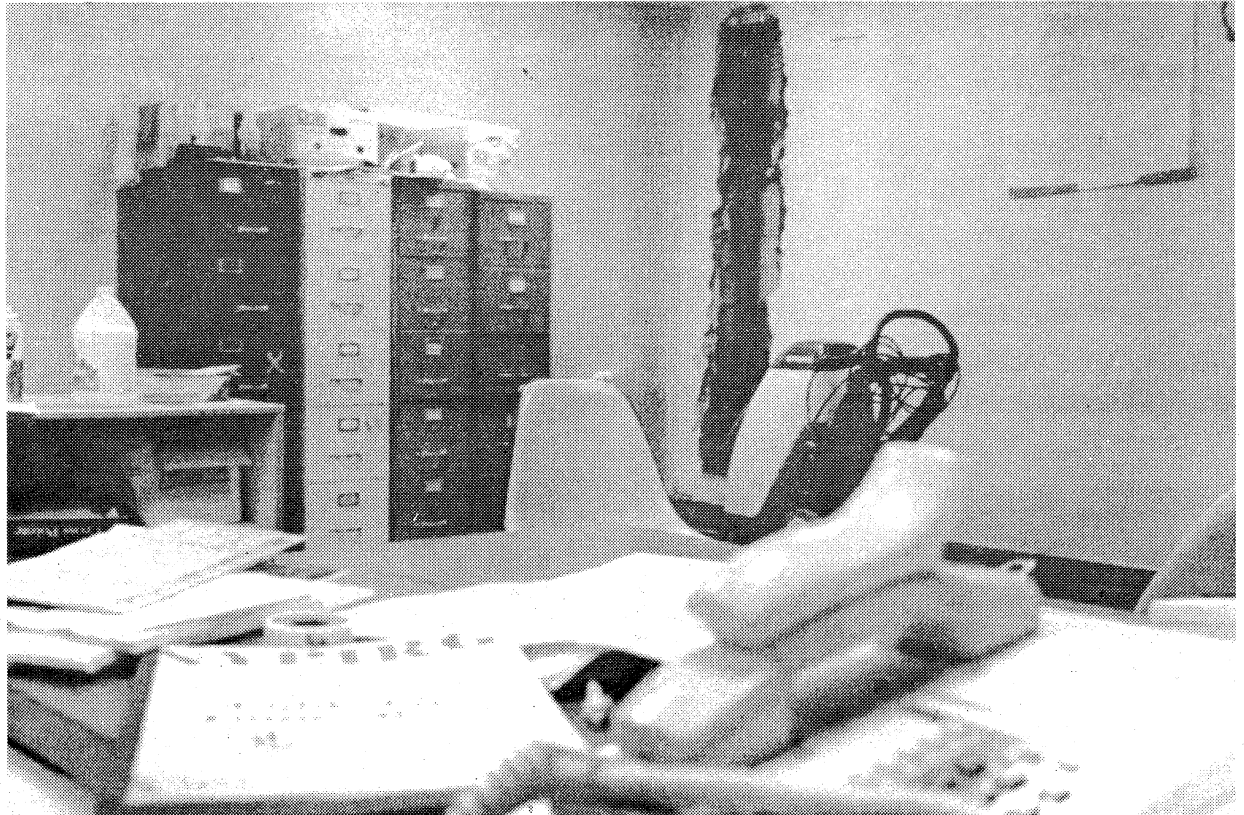
The NYPIRG office has runoff waste leaking into the room.
