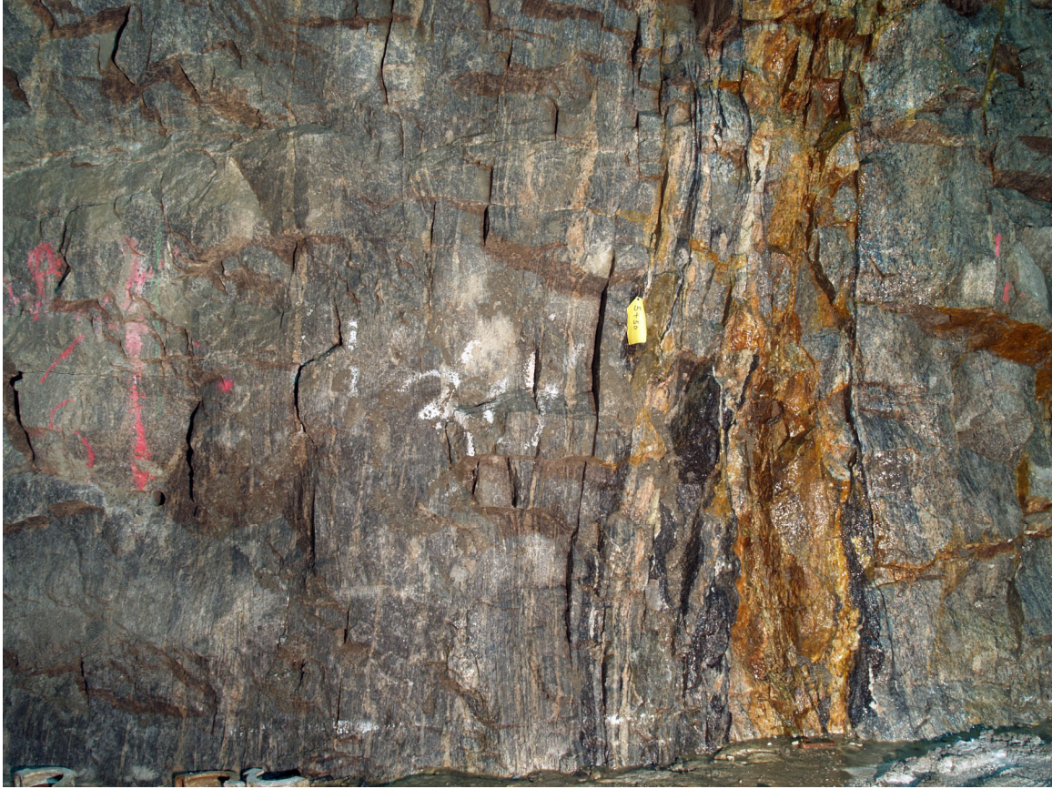
Figure 7 - Typical Yonkers Gneiss (Zy). Station 5+50, north wall raw water tunnel, Croton Water Treatment Plant, Bronx, New York. (Digital image by C. Merguerian).
