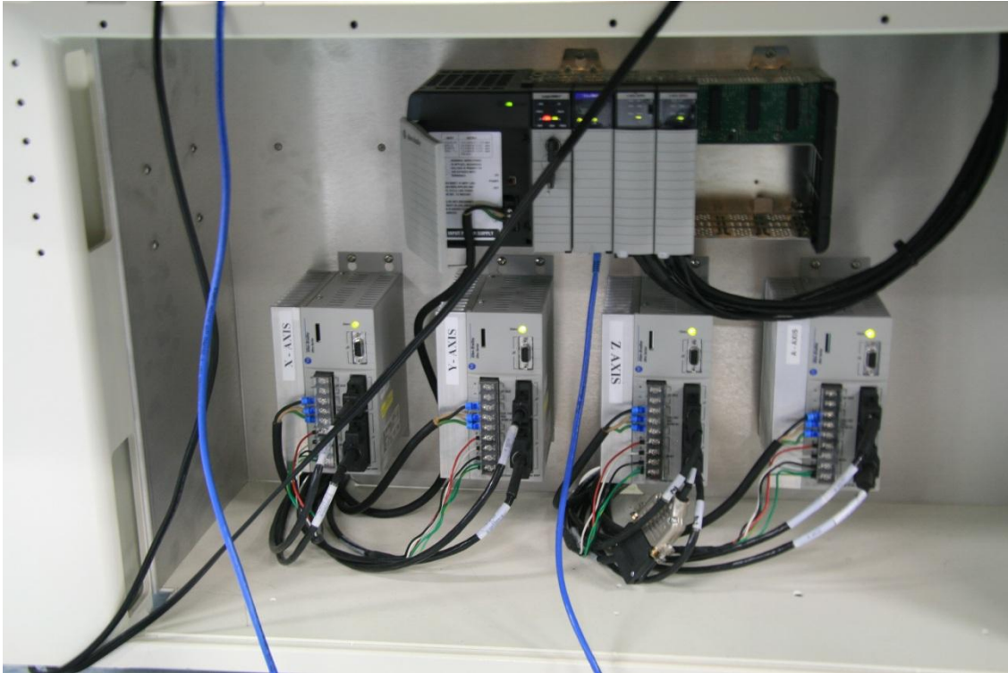
Figure 3-3: Servo and Controller Setup
