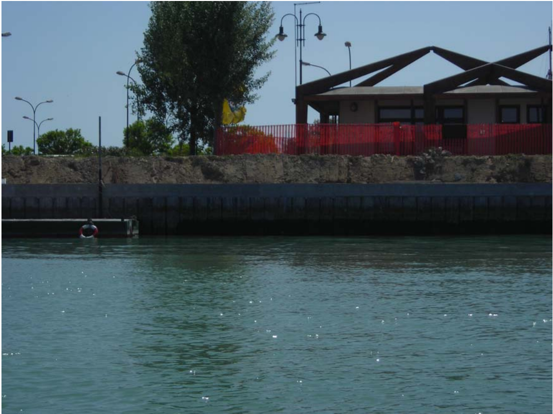
Figure 2. Photo of the construction work at the new marina near Treporti. Previously, this was a gently sloping hill with a small sandy beach back towards the building.
