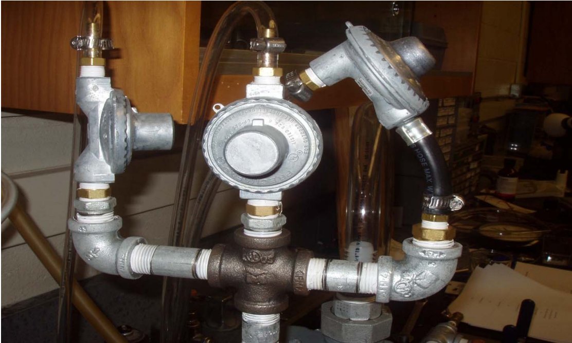
Figure 10. Three propane regulators at inlet of gas meter
