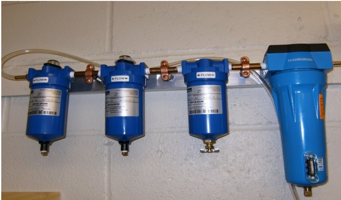
Figure 8. Filters - particle, oil, coalescing and desiccant
