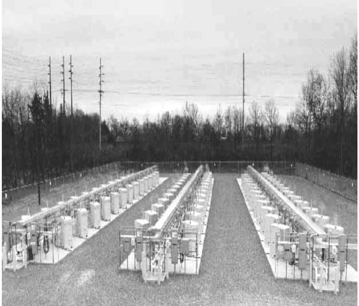
Figure 1. 8 Fuel cell substation in West Babylon, NY as a part of LIPA's fuel cell substation with 3 rows of 25 grid connected fuel cells [4].
