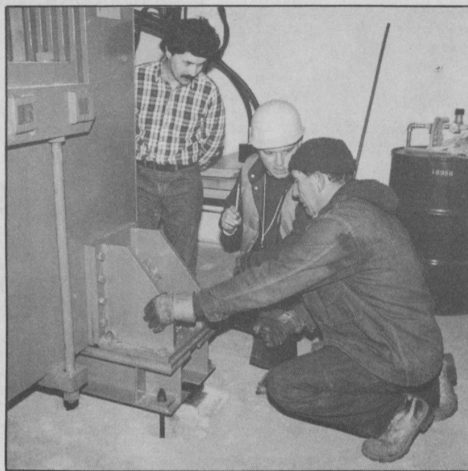
4. As crew completes attachment of machine to floor base, Liebermann discusses the process of leveling with a worker. Research associate Tibor Gasparik looks on.
