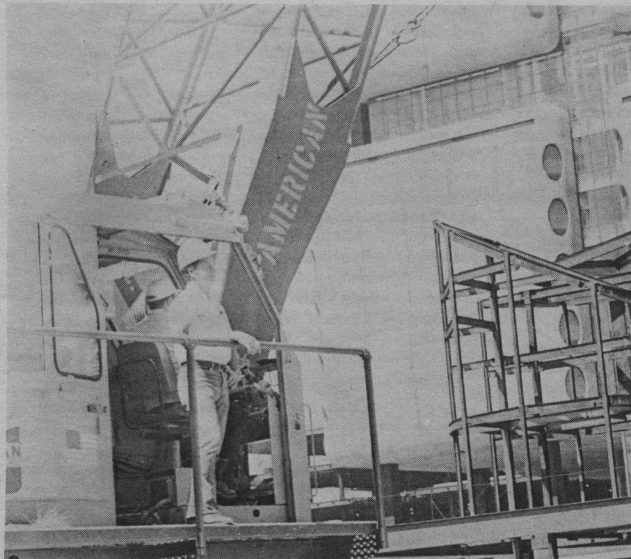
AL BRISKIE in his hard hat, on the job, surveys the new HSC building. photo by Toni Bosco
