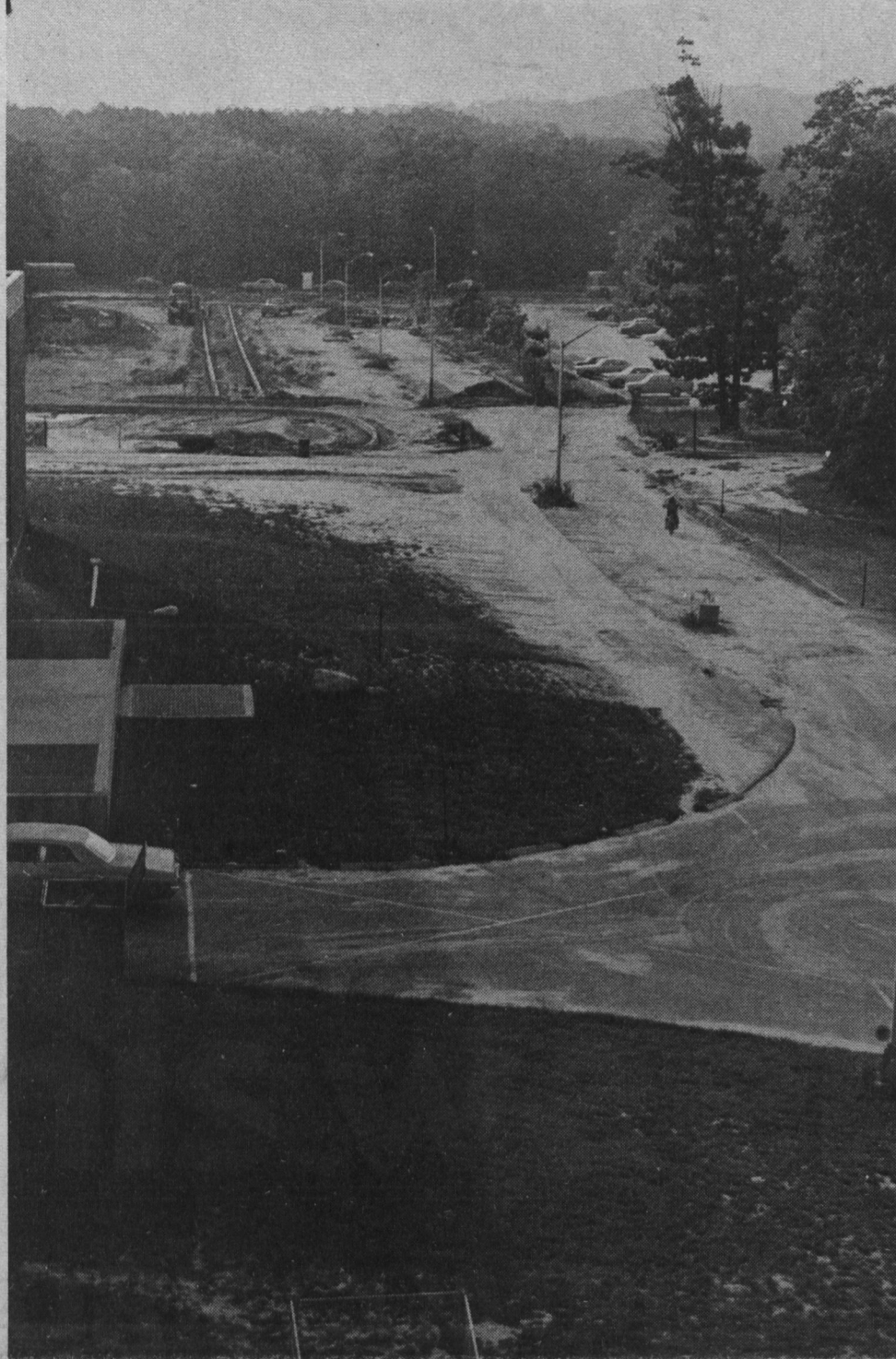
North ESS Lot, which can be seen in the background, has been completed.
