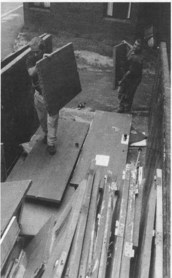
Renhabbing of Kelly Quad is underway. Here workmen remove old interior doors
