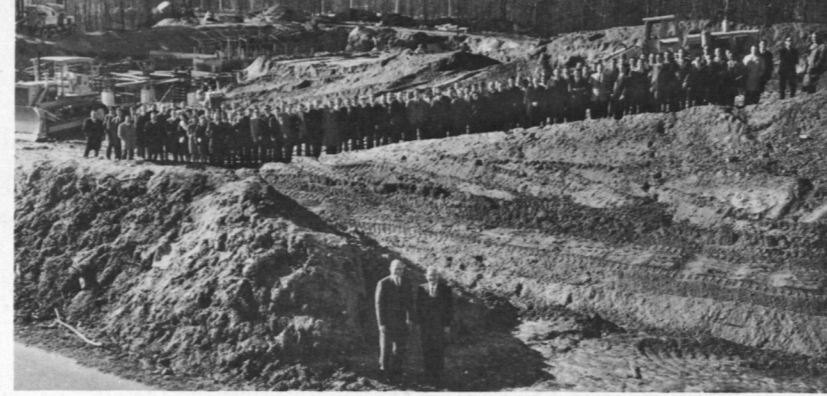
The growth of the campus has meant much watching (above, President John S. Toll, Academic Vice President Bentley Glass and faculty members view early days in the construction of the earth and space sciences building, shown completed below) and waiting (right).
