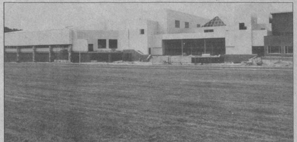
Construction of the new Stony Brook Indoor Athletic Complex, which features a 4,100 seat arena, indoor track, squash courts and locker room facilities, is scheduled to be completed this fall.
