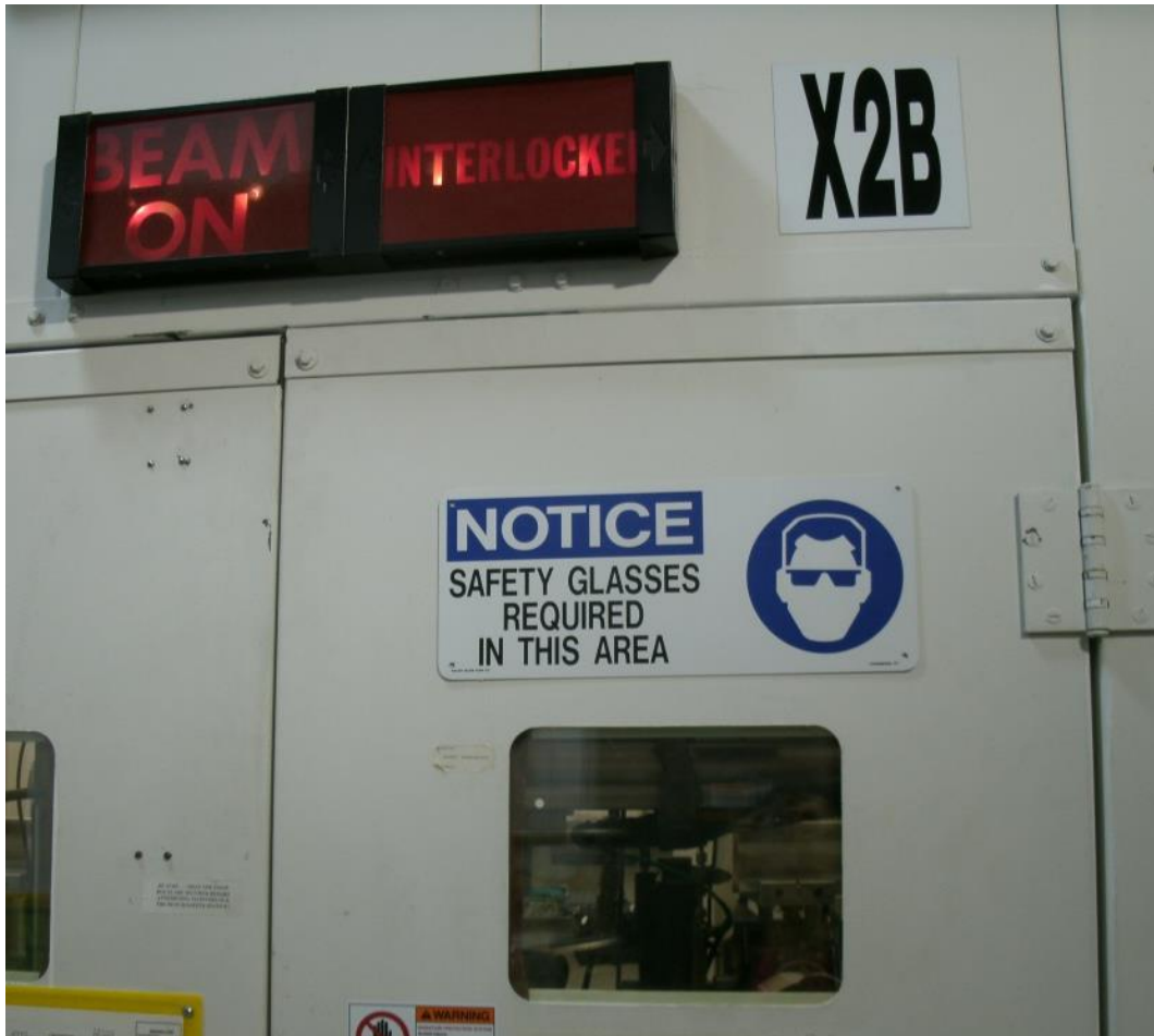
Figure 2.10: Interlock and Beam On indicator lights above the experimental hutch doors
