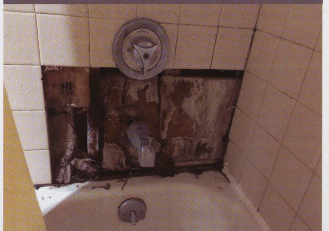
A resident of West Apartments B, who wished not to be named for her connection to campus residences, lived in his room all summer with a shower that looked like this. It wasn't fixed by the beginning of the 2015 Fall semester but was fixed about two weeks in.
