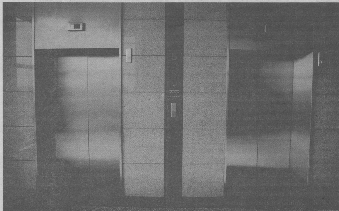
Two elevators in a building. Elevators are cramped spaces that can bring about a number of issues for the people inside them.
