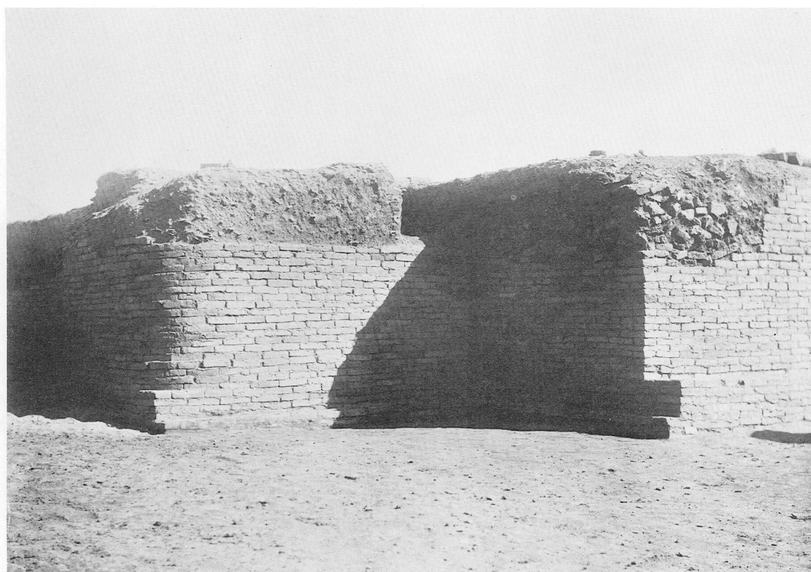
(b) The outer face at the west corner, shewing rounded brickwork. (p. 30)
