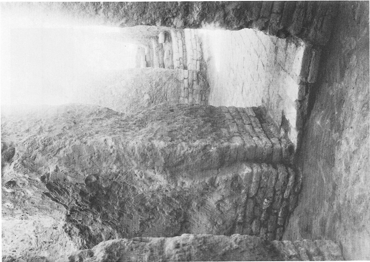
a. No. 11 Paternoster Row; view from Room 6 to the secondary front door 11b
