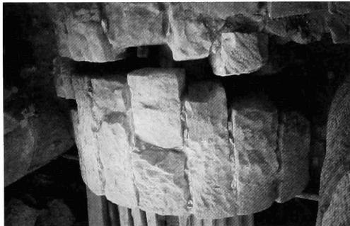
Figure 2.80. Arched doorway, West Corridor, requiring consolidation, 1997.
