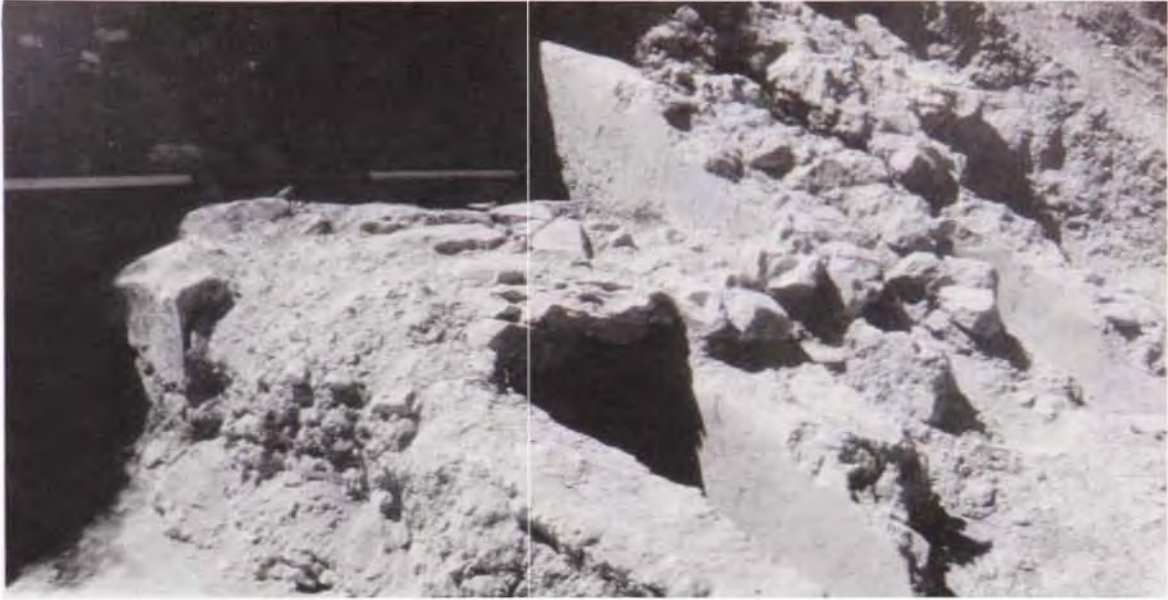
Fig. 4.24. Site E1: channels excavated. Channel 3 is in foreground. Note plastered wall of Channel 2 behind.
