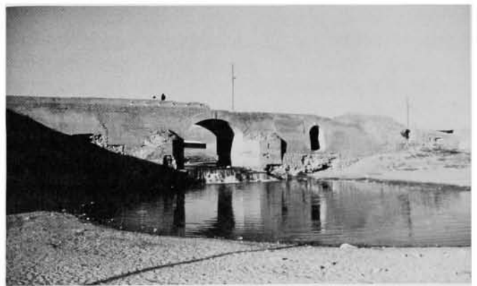
FIG. 30. Bridge over the Ab-i Marik at Mahidasht village, showing mid-17th century A.D. foundations buried by alluvial Units IVb–II, partially re-exposed by recent stream incision. 11 July 1978.
