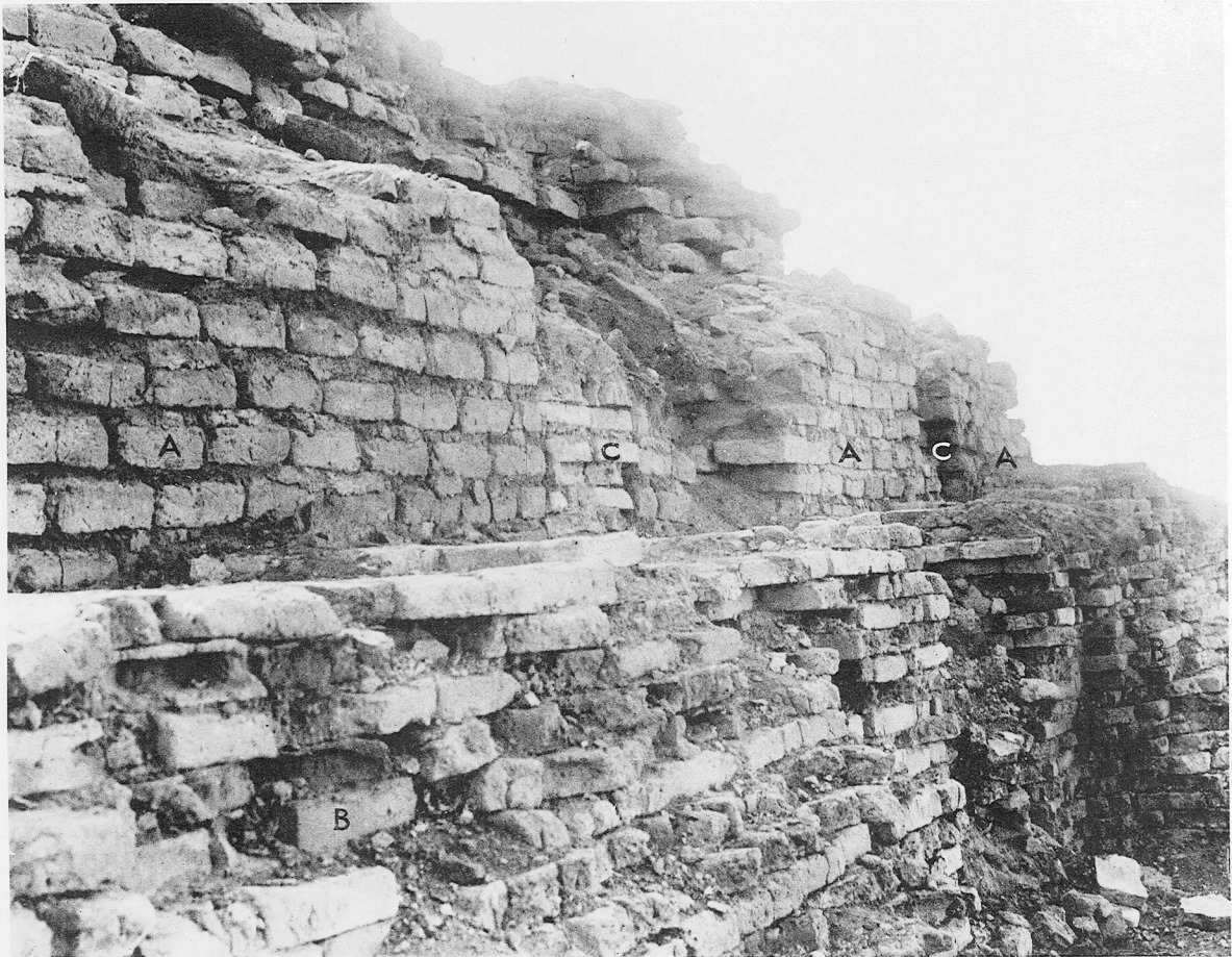
a. The NW. side of the Ziggurat, upper terrace: A . . . A, the crude brick core of the Nabonidus upper story; B . . . B, remains of burnt-brick casing; c, c, burnt-brick keys inset in the mud-brickwork. (See p. 127)
